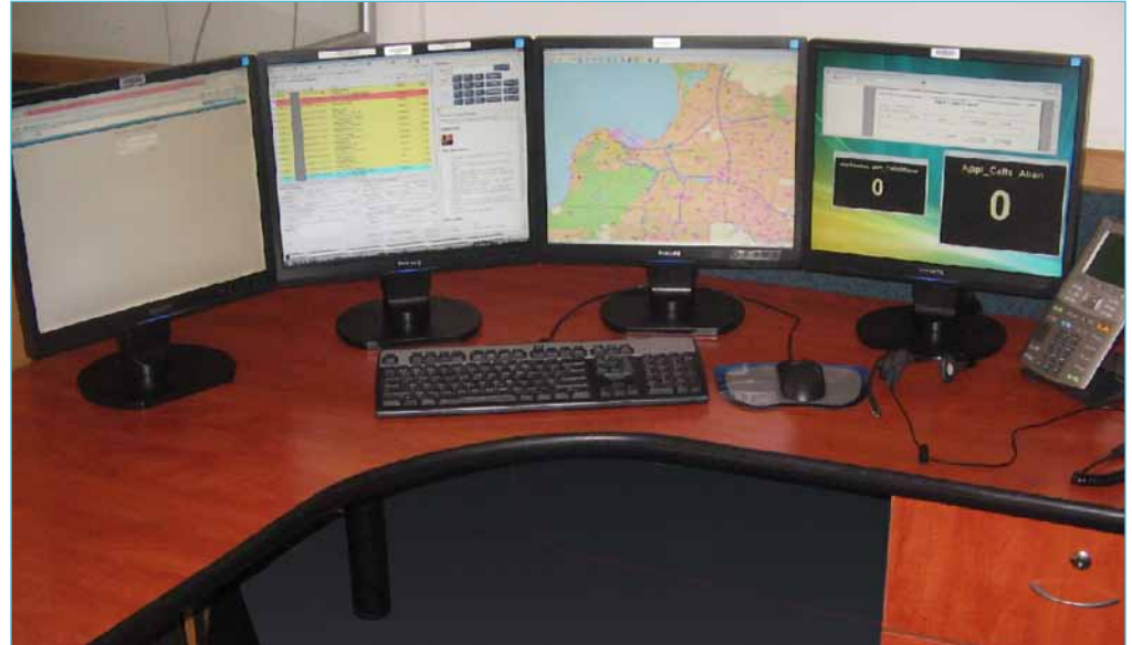
Matrox Extio F1400 units drive four-monitor emergency service operator stations at 1-0-7 Emergency
